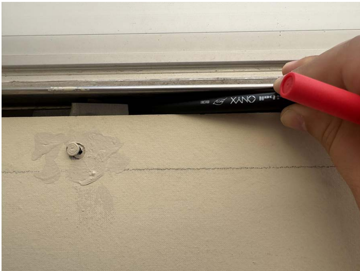
REPLACE DAMAGED, WARPED AND MISSING SIDING
