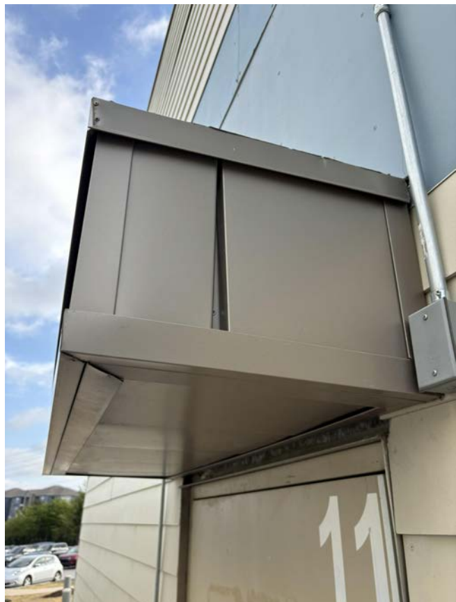
METAL PANEL ON CANOPY TO BE REALIGNED
