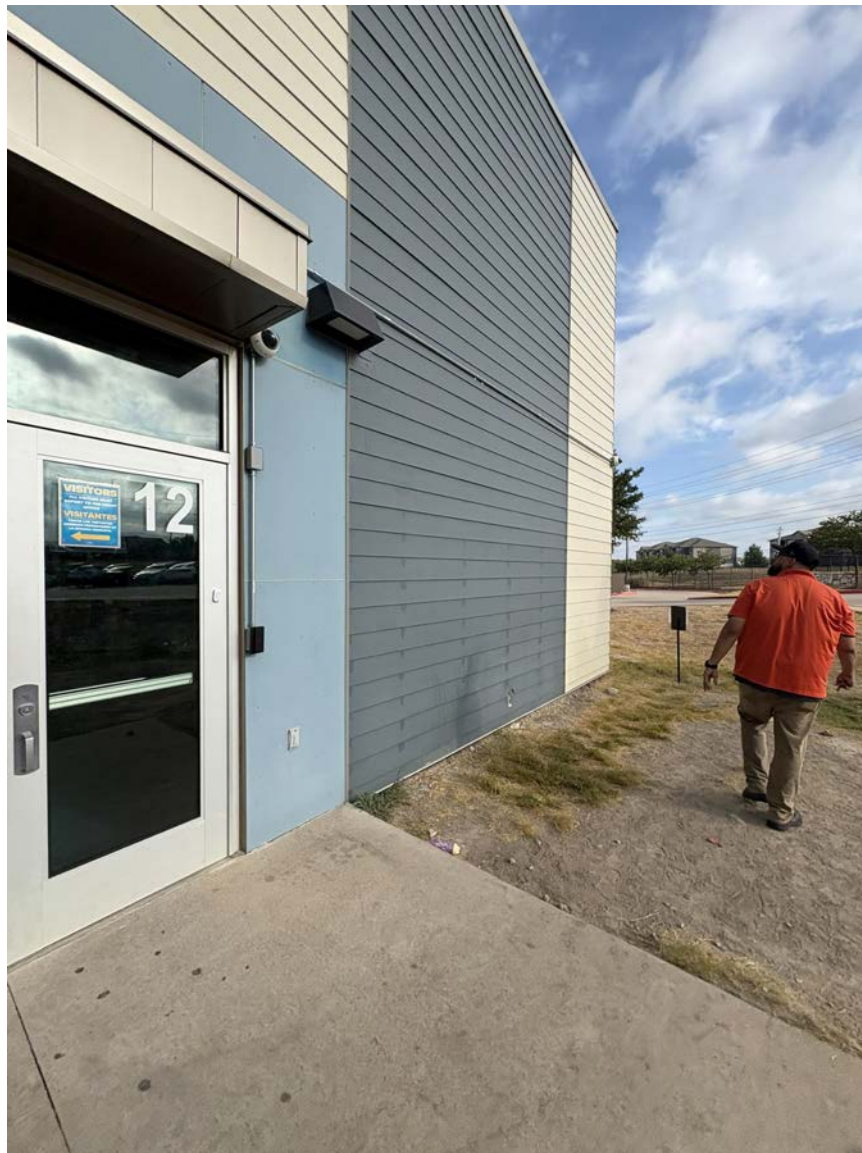
REPLACE DAMAGED, WARPED AND MISSING SIDING
