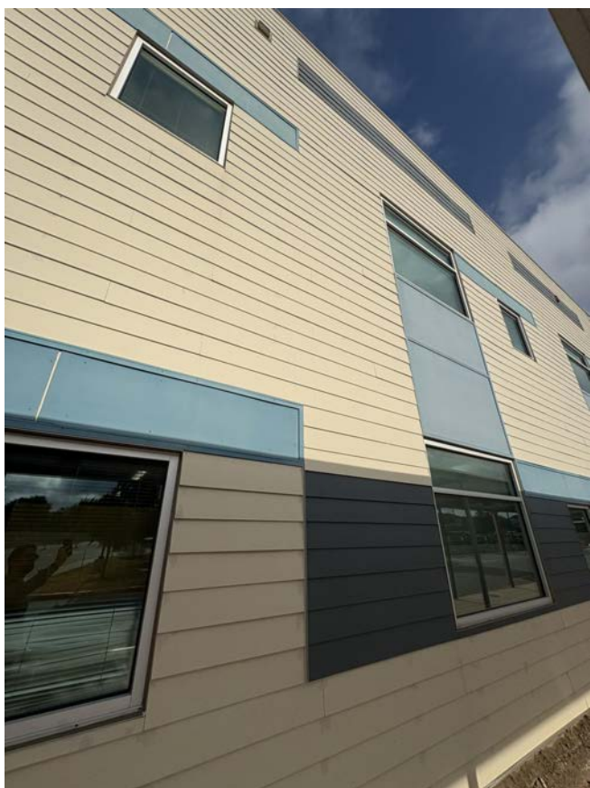
REPLACE DAMAGED, WARPED AND MISSING SIDING
