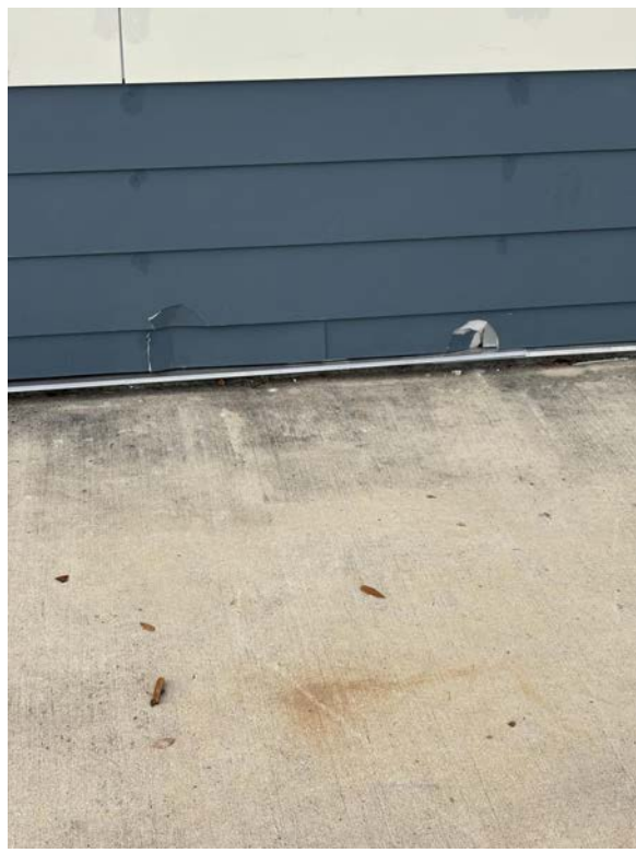
REPLACE DAMAGED, WARPED AND MISSING SIDING
