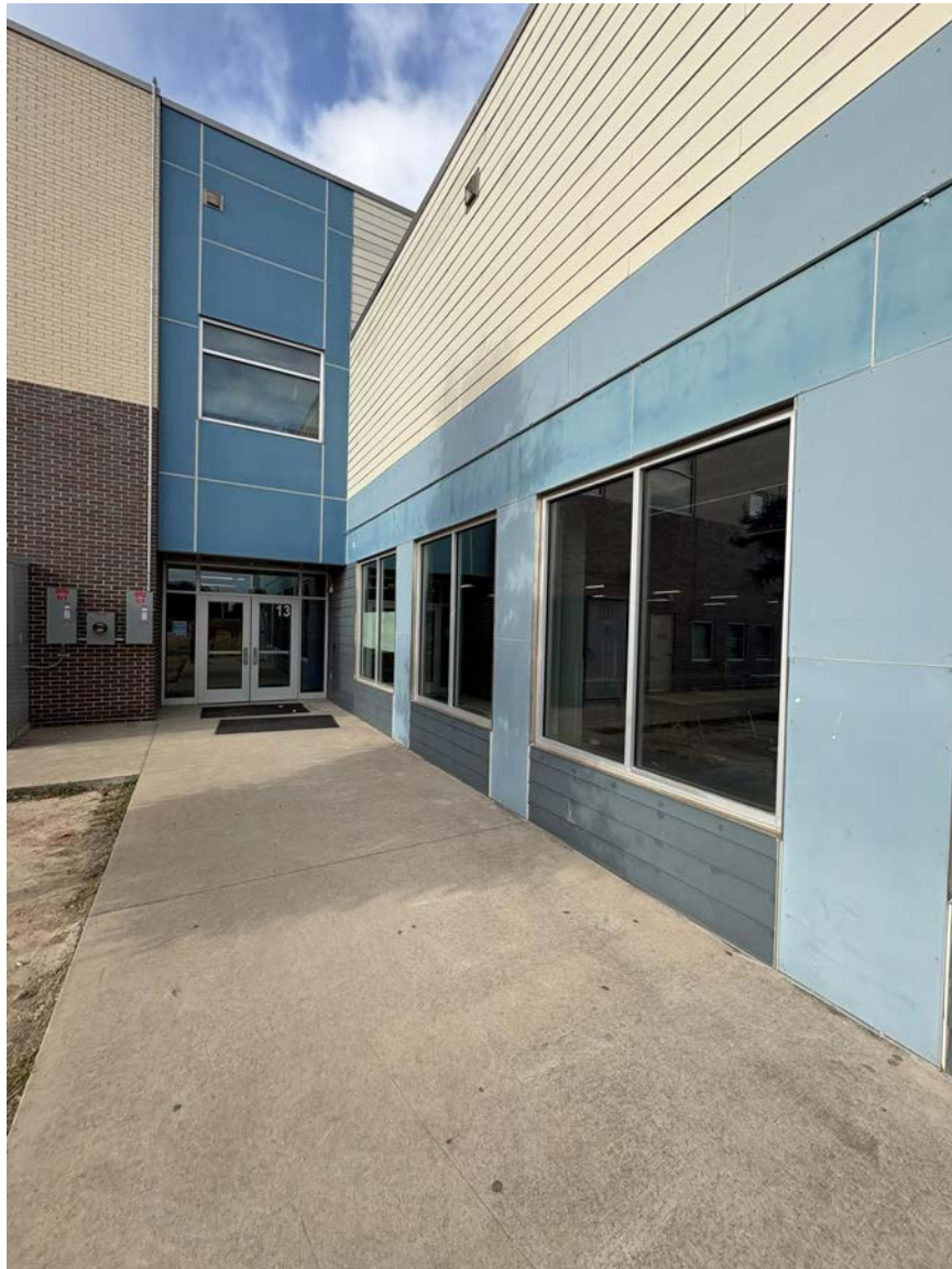
REPLACE DAMAGED, WARPED AND MISSING SIDING
