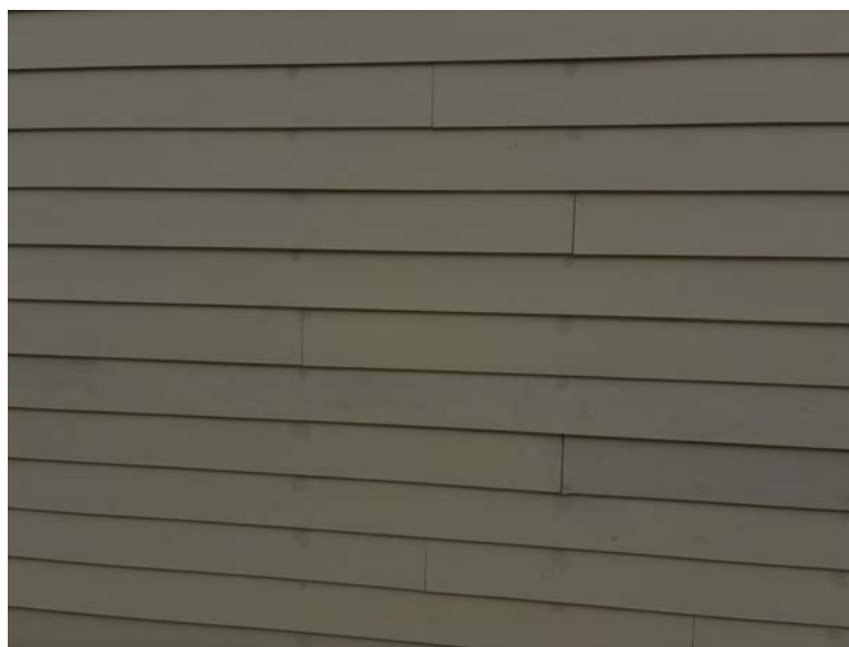
REPLACE DAMAGED, WARPED SIDING
