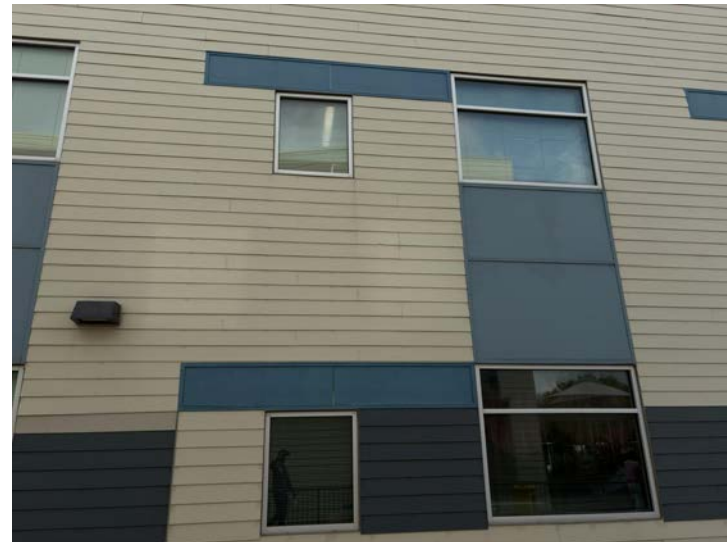
REPLACE DAMAGED, WARPED AND MISSING SIDING
