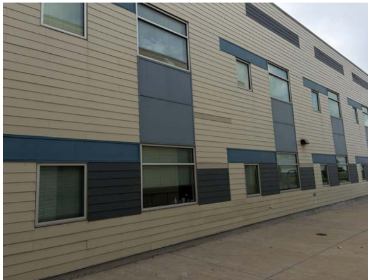
REPLACE DAMAGED, WARPED AND MISSING SIDING
