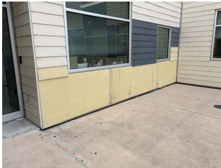
REPLACE MISSING SIDING
