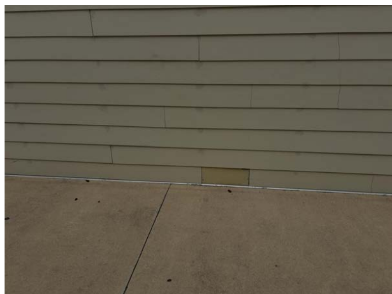
REPLACE DAMAGED, WARPED AND MISSING SIDING
