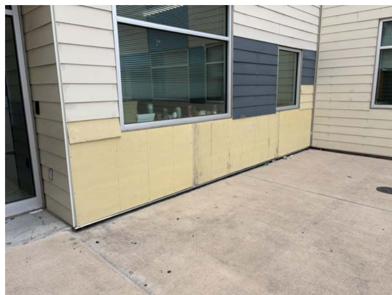
REPLACE DAMAGED, WARPED AND MISSING SIDING
