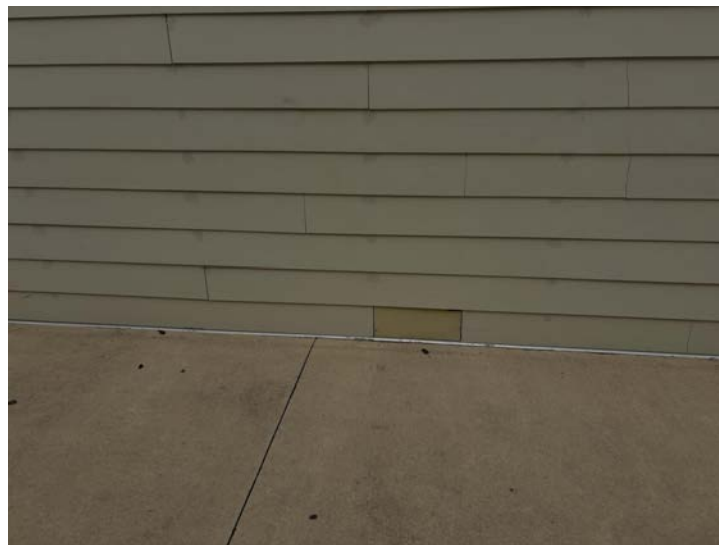
REPLACE MISSING SIDING
