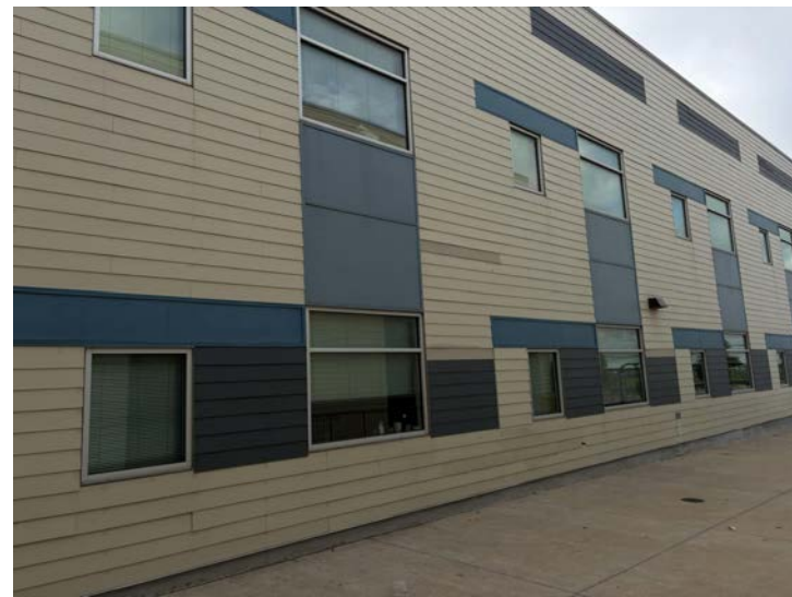
REPLACE DAMAGED, WARPED AND MISSING SIDING
