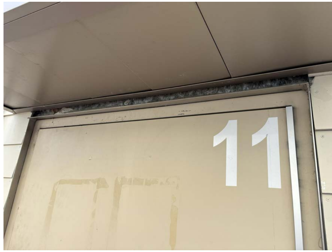
METAL PANEL ON CANOPY TO BE REALIGNED
