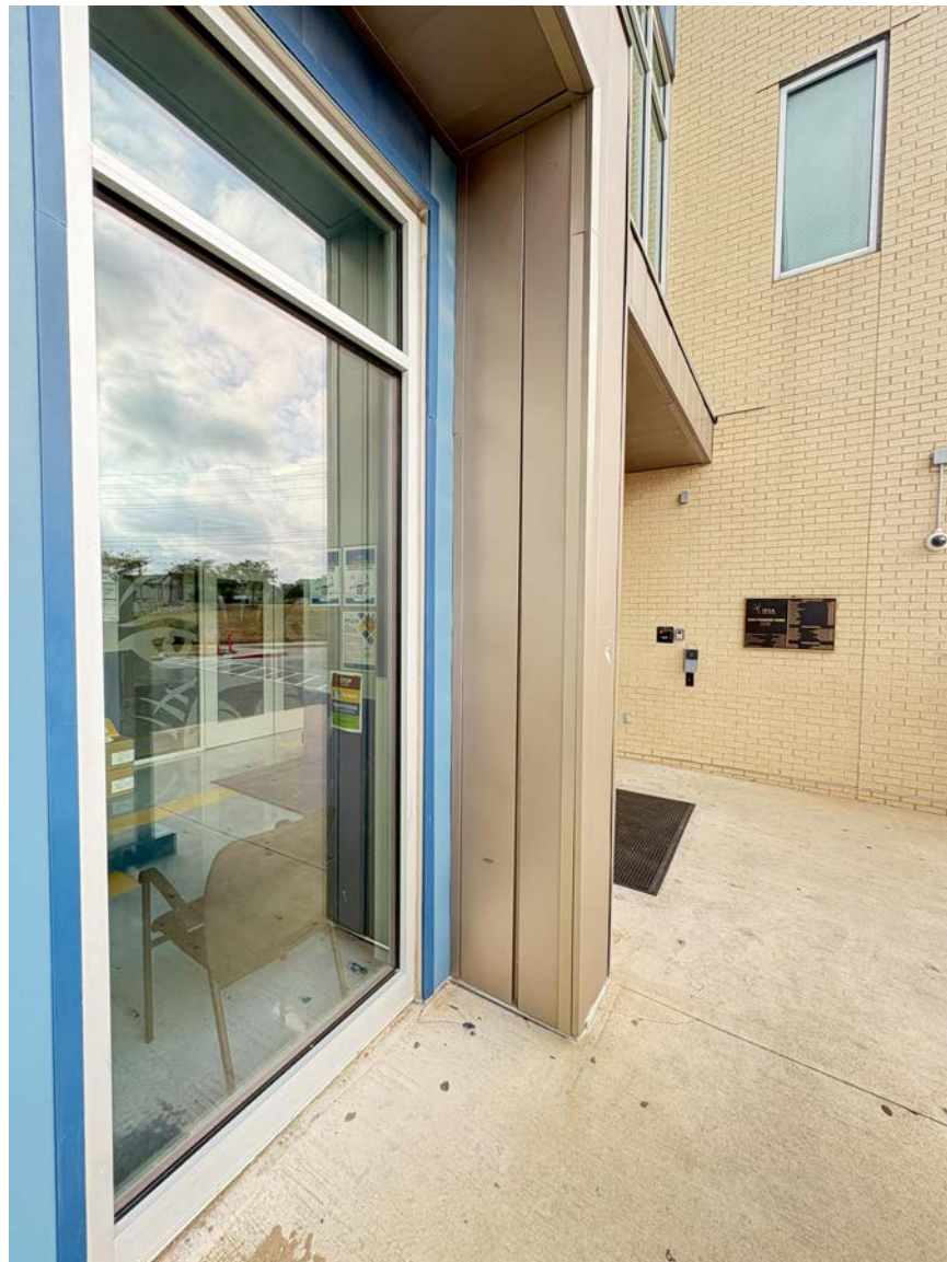
METAL PANEL ON FUR OUT TO BE REALIGNED
