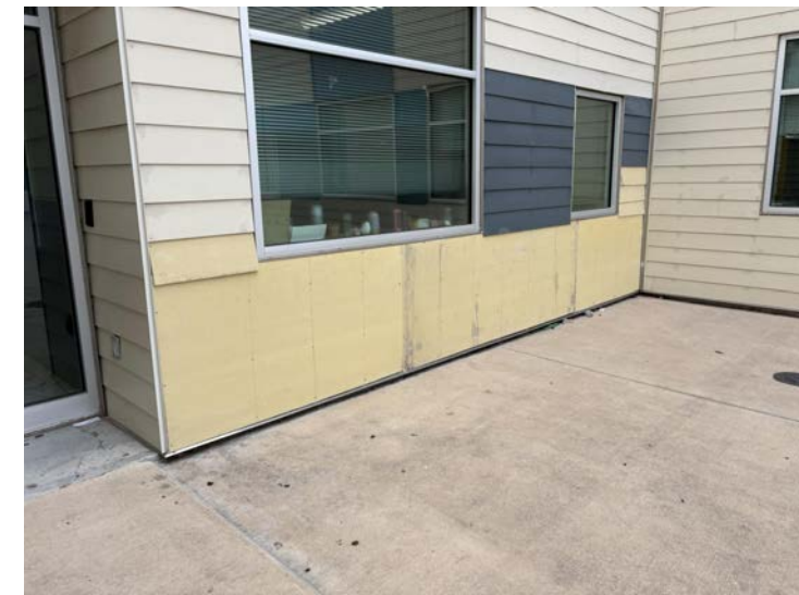
REPLACE MISSING SIDING
