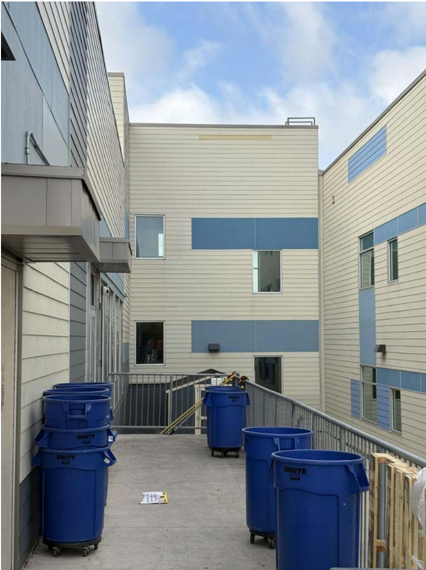
REPLACE DAMAGED, WARPED AND MISSING SIDING
