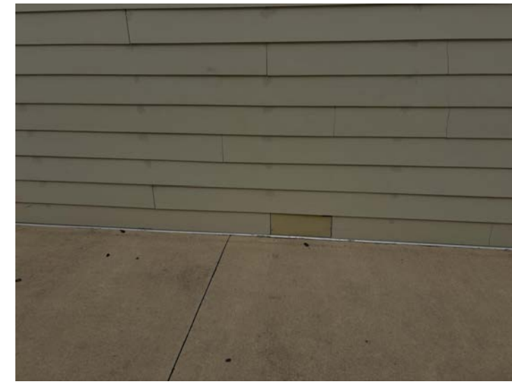
REPLACE MISSING SIDING
