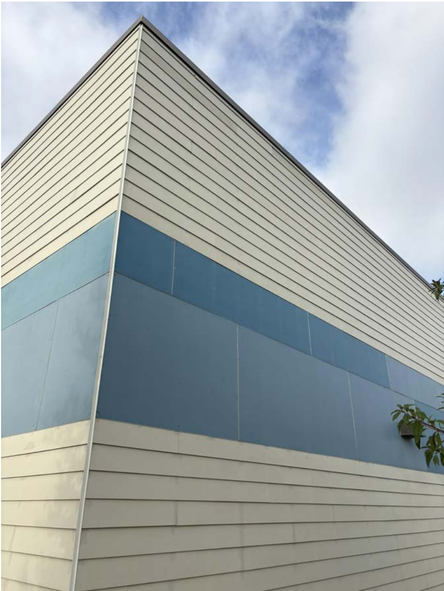
REPLACE DAMAGED AND MISSING SIDING
