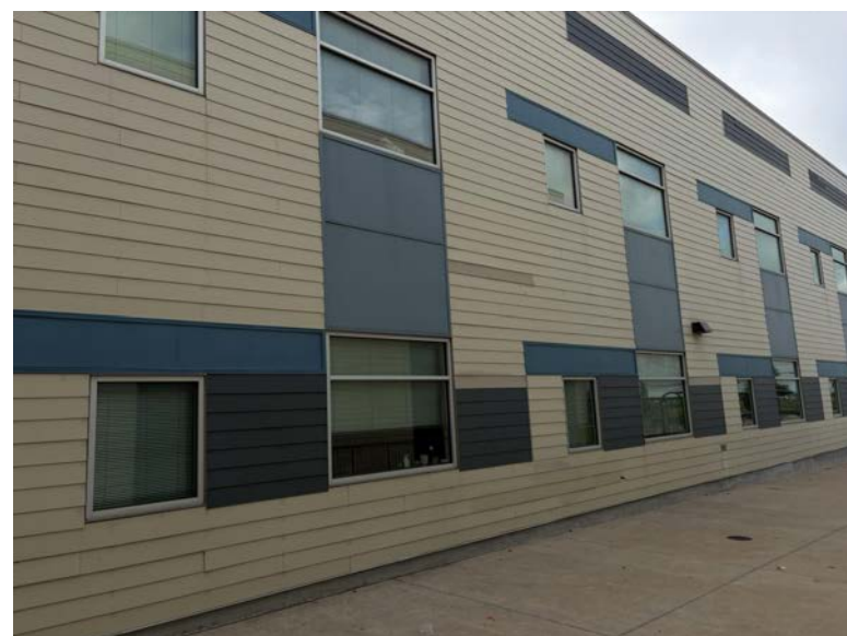
REPLACE DAMAGED, WARPED AND MISSING SIDING
