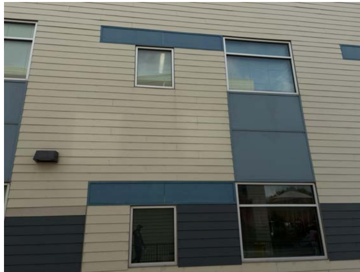
REPLACE DAMAGED, WARPED AND MISSING SIDING
