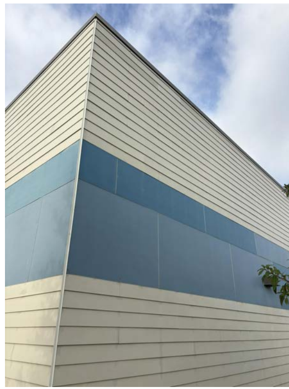
REPLACE DAMAGED, WARPED AND MISSING SIDING
