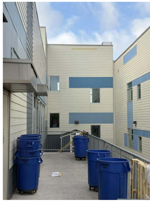
REPLACE DAMAGED, WARPED AND MISSING SIDING
