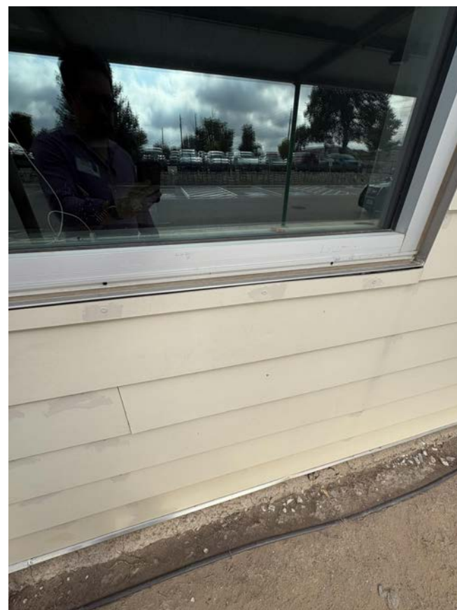
REPLACE DAMAGED, WARPED SIDING
