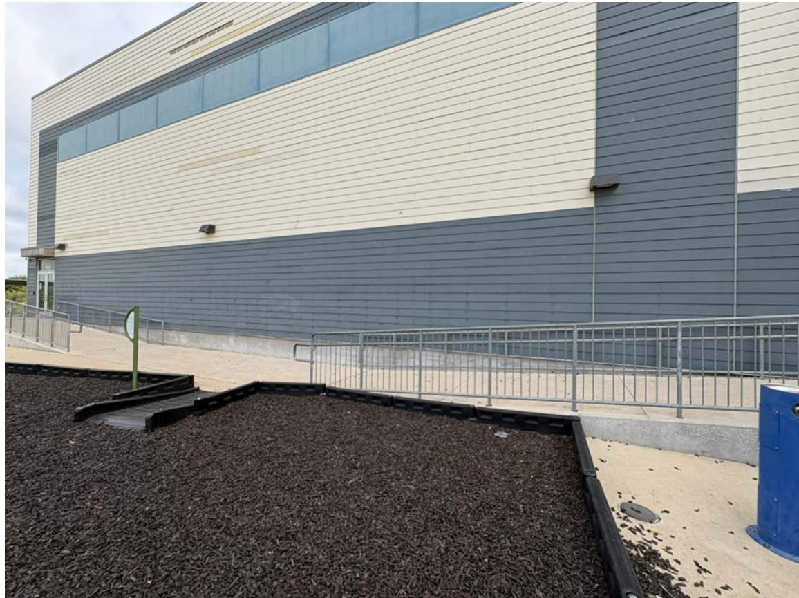
REPLACE DAMAGED, WARPED AND MISSING SIDING
