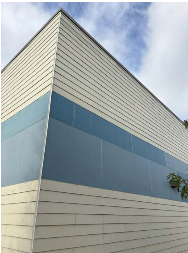
REPLACE DAMAGED, WARPED AND MISSING SIDING
