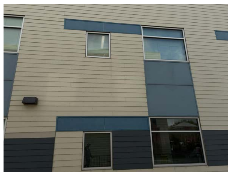
REPLACE DAMAGED, WARPED AND MISSING SIDING
