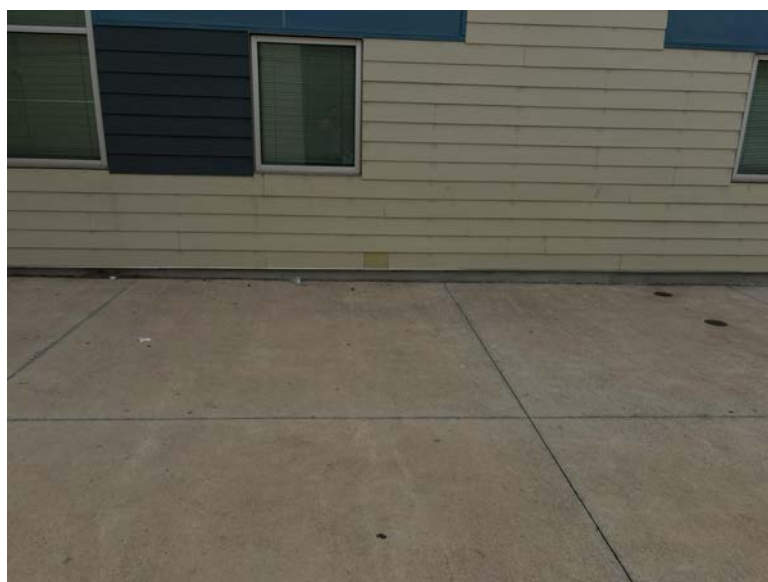
REPLACE DAMAGED, WARPED AND MISSING SIDING
