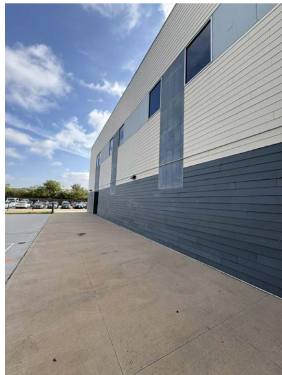
REPLACE DAMAGED AND WARPED SIDING.
