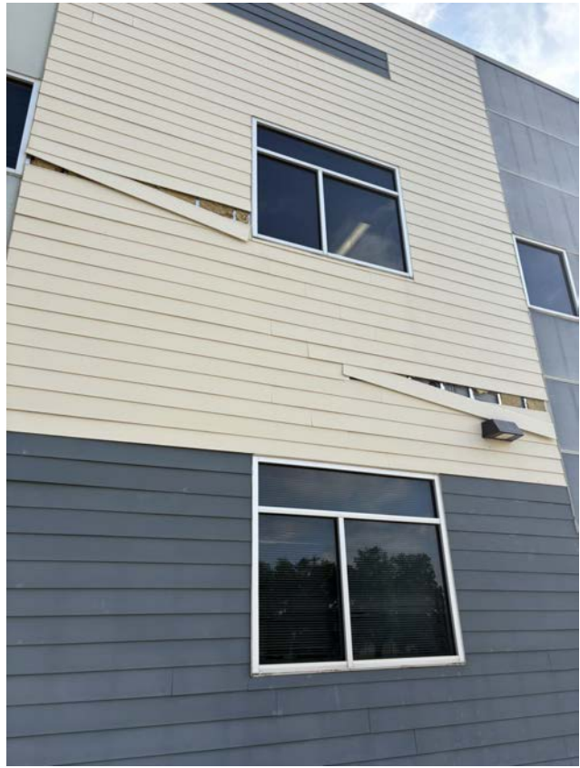
REPLACE DAMAGED SIDING
