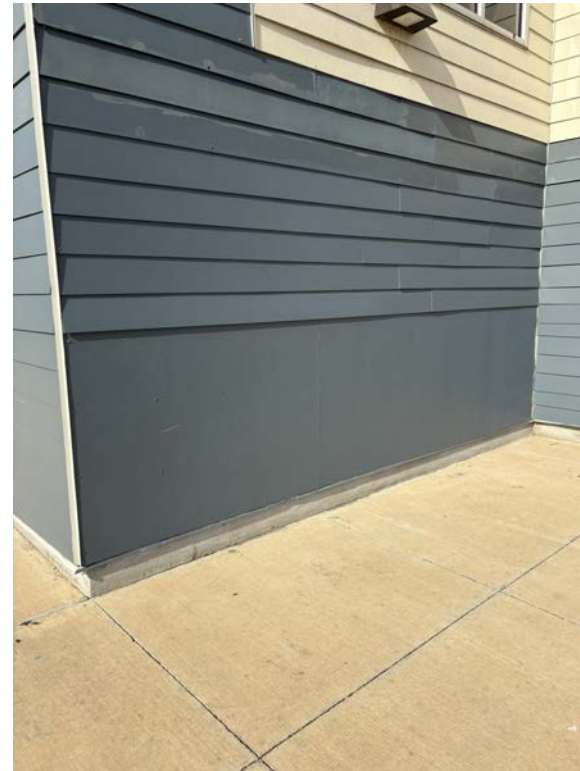
REPLACE DAMAGED AND WARPED SIDING.
