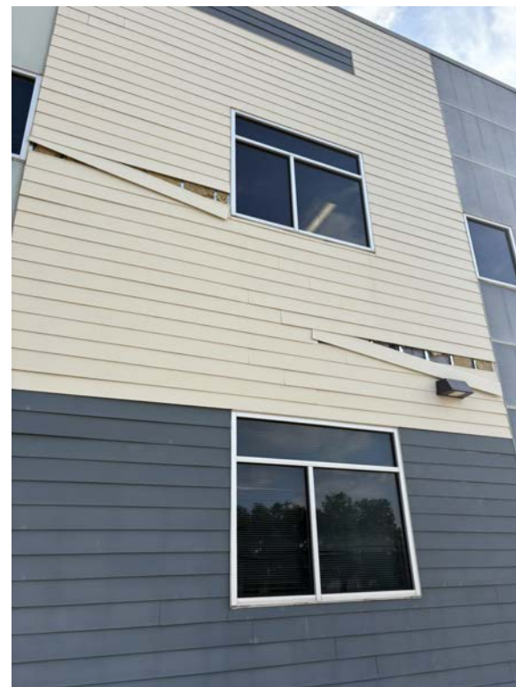
REPLACE DAMAGED, MISSING, AND WARPED SIDING.
