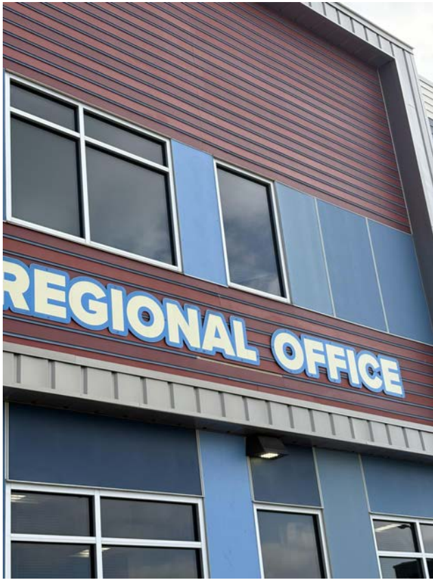
REPLACE MISSING SIDING
