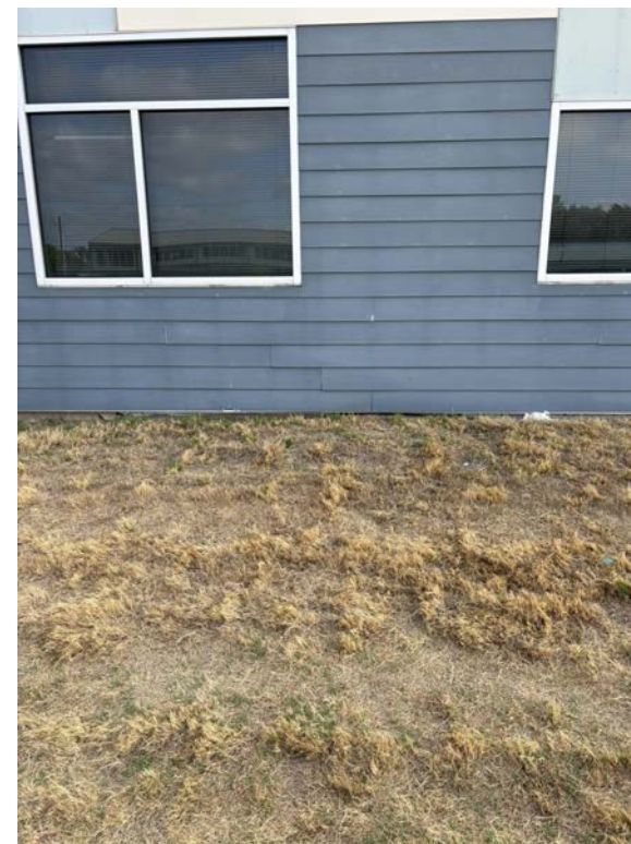
REPLACE DAMAGED AND WARPED SIDING.
