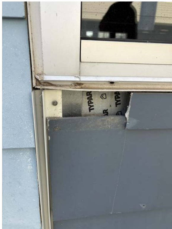
REPLACE DAMAGED AND WARPED SIDING.
