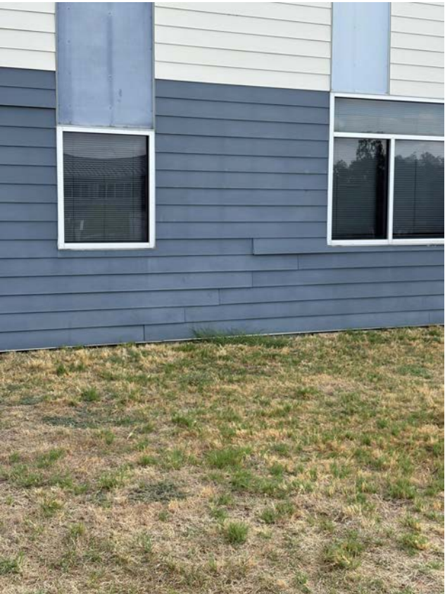
REPLACE MISSING SIDING
