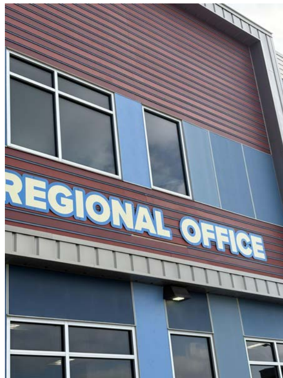
REPLACE DAMAGED, MISSING, AND WARPED SIDING.
