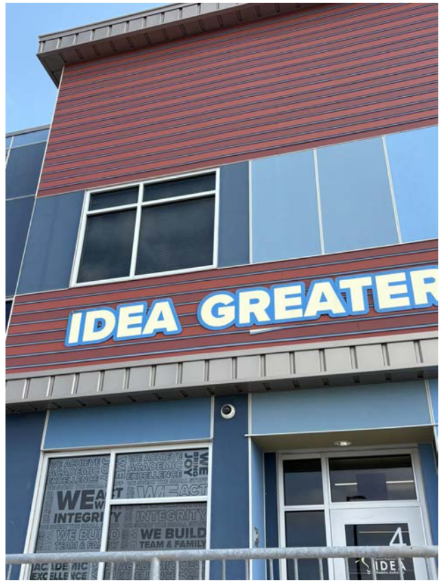
REPLACE DAMAGED SIDING
