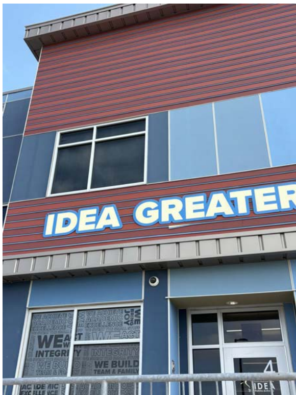
REPLACE DAMAGED, MISSING, AND WARPED SIDING.
