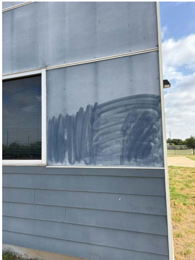
REPLACE DAMAGED SIDING
