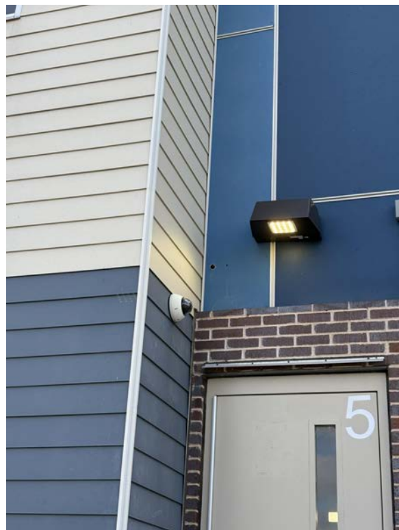
REPLACE DAMAGED SIDING
