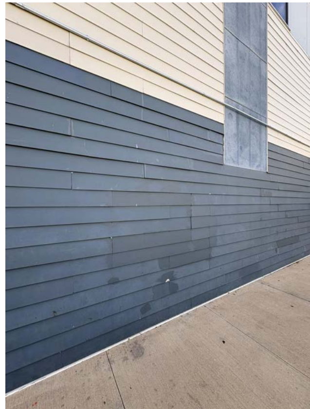
REPLACE DAMAGED SIDING
