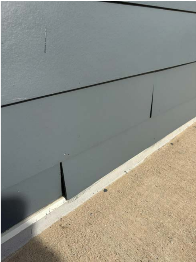
REPLACE DAMAGED SIDING
