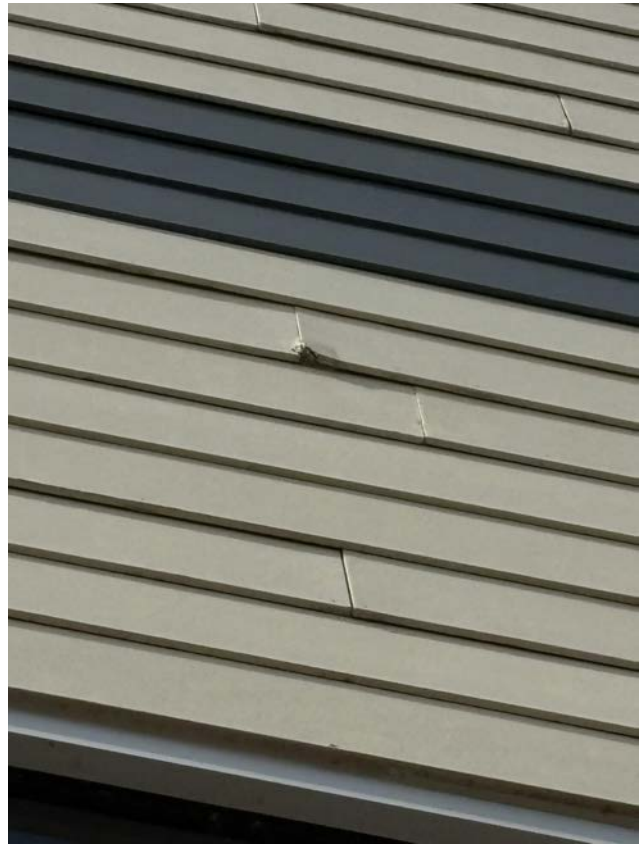
REPLACE DAMAGED SIDING
