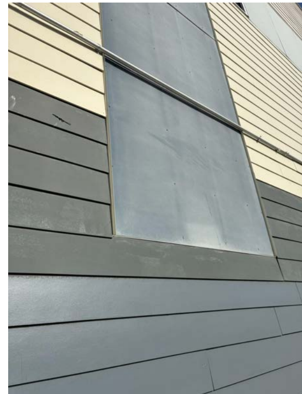
REPLACE DAMAGED SIDING.
