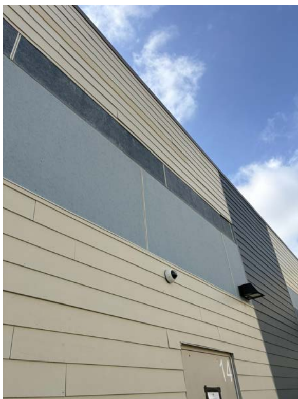
REPLACE DAMAGED AND WARPED SIDING.
