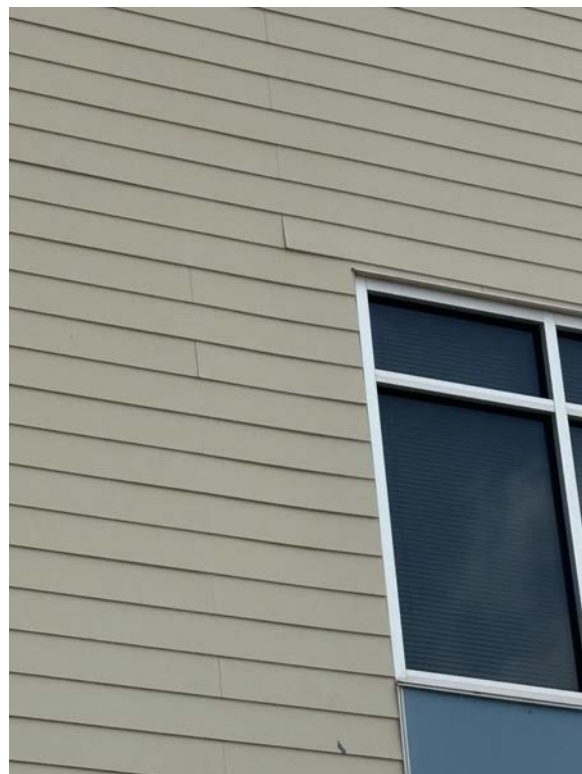
REPLACE DAMAGED AND WARPED SIDING.
