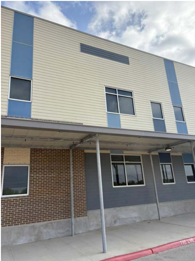
REPLACE DAMAGED AND WARPED SIDING
