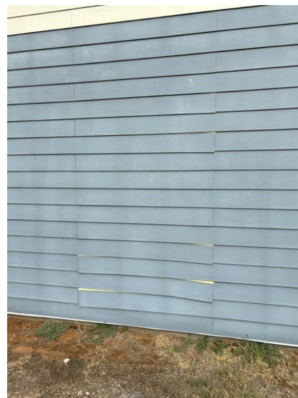
REPLACE DAMAGED SIDING.
