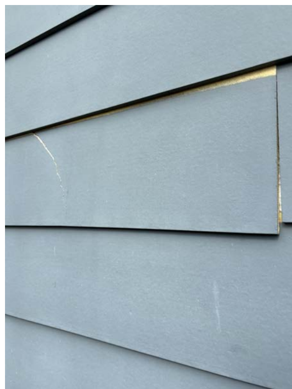
REPLACE DAMAGED AND WARPED SIDING.
