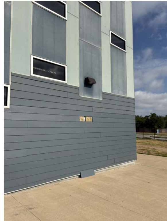
REPLACE DAMAGED, MISSING, AND WARPED SIDING.
