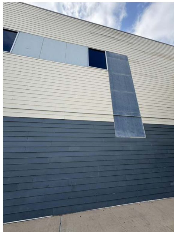
REPLACE DAMAGED AND WARPED SIDING.
