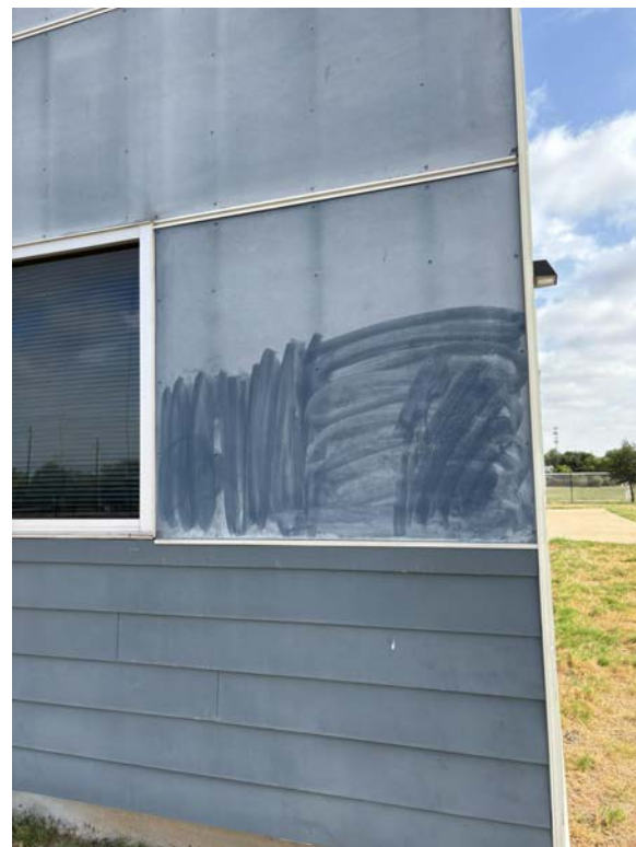
REPLACE DAMAGED SIDING.
