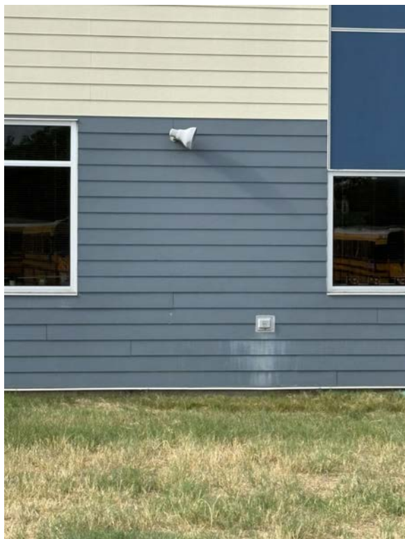
REPLACE DAMAGED SIDING.
