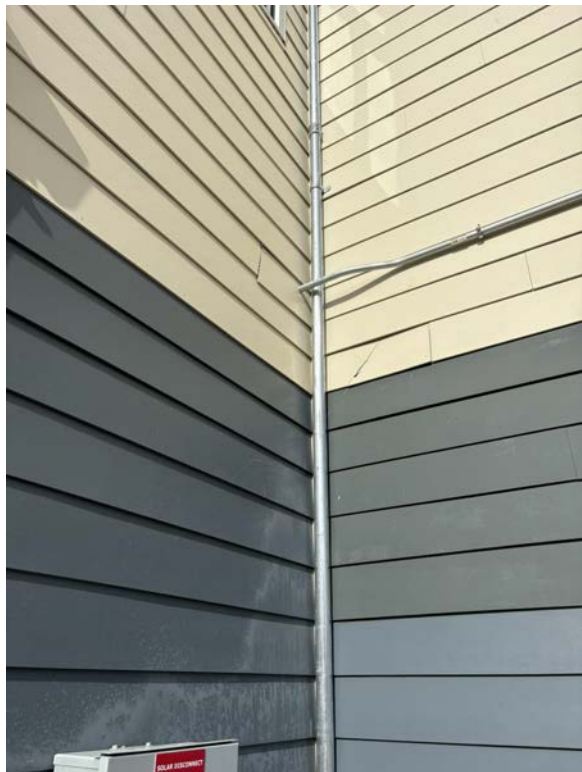
REPLACE DAMAGED AND WARPED SIDING.
