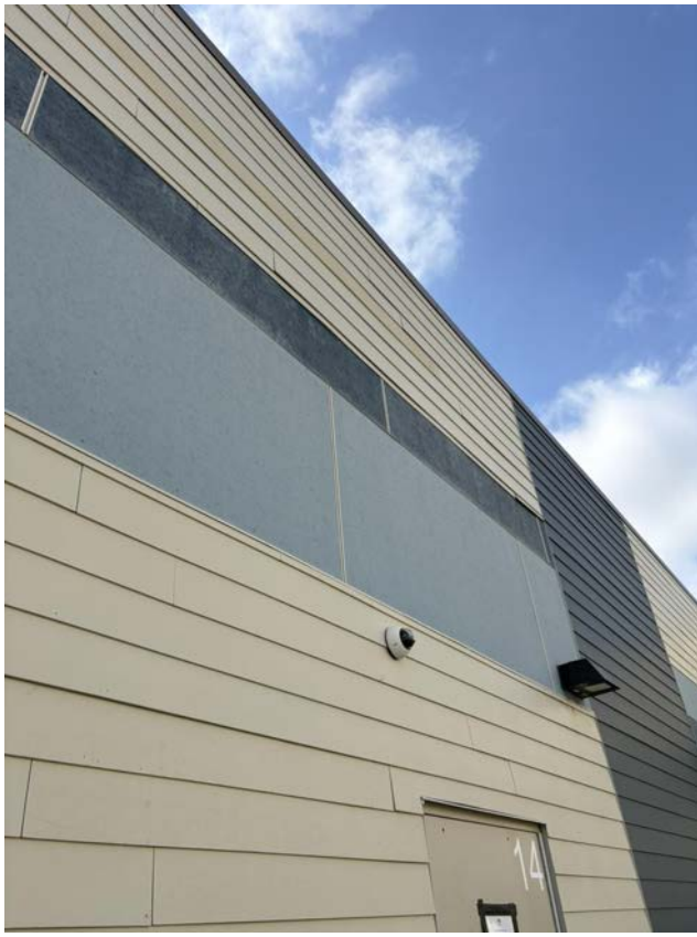
REPLACE DAMAGED SIDING
