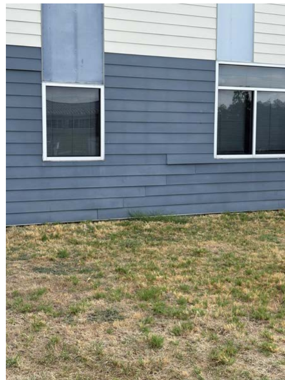
REPLACE DAMAGED AND WARPED SIDING.
