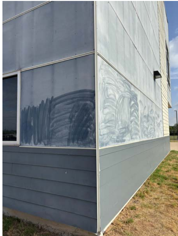
REPLACE DAMAGED SIDING.
