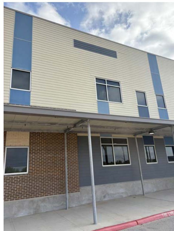
REPLACE DAMAGED, MISSING, AND WARPED SIDING.
