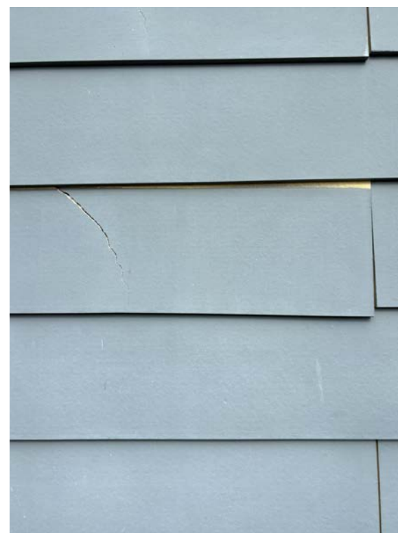
REPLACE DAMAGED SIDING.
