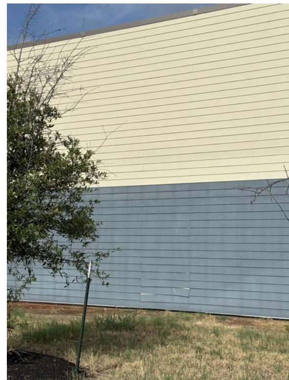
REPLACE DAMAGED SIDING.
