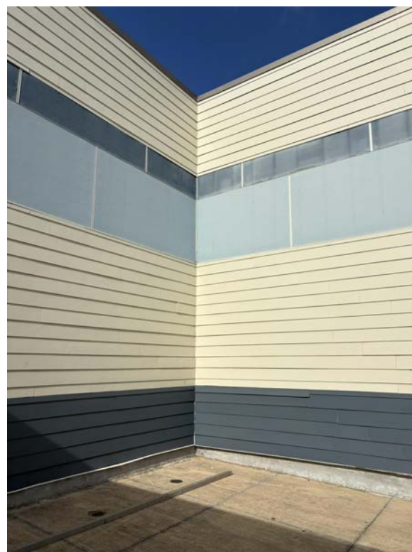
REPLACE DAMAGED SIDING.
