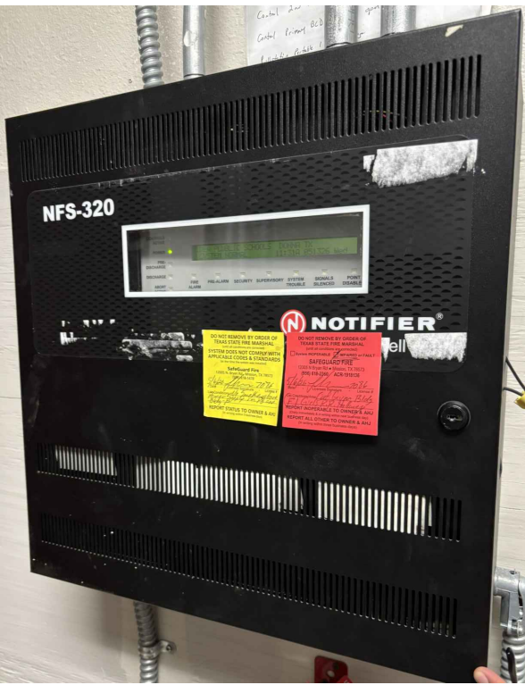
01 EXISTING FIRE ALARM CONTROL PANEL IMAGE SCALE : NOT TO SCALE.
