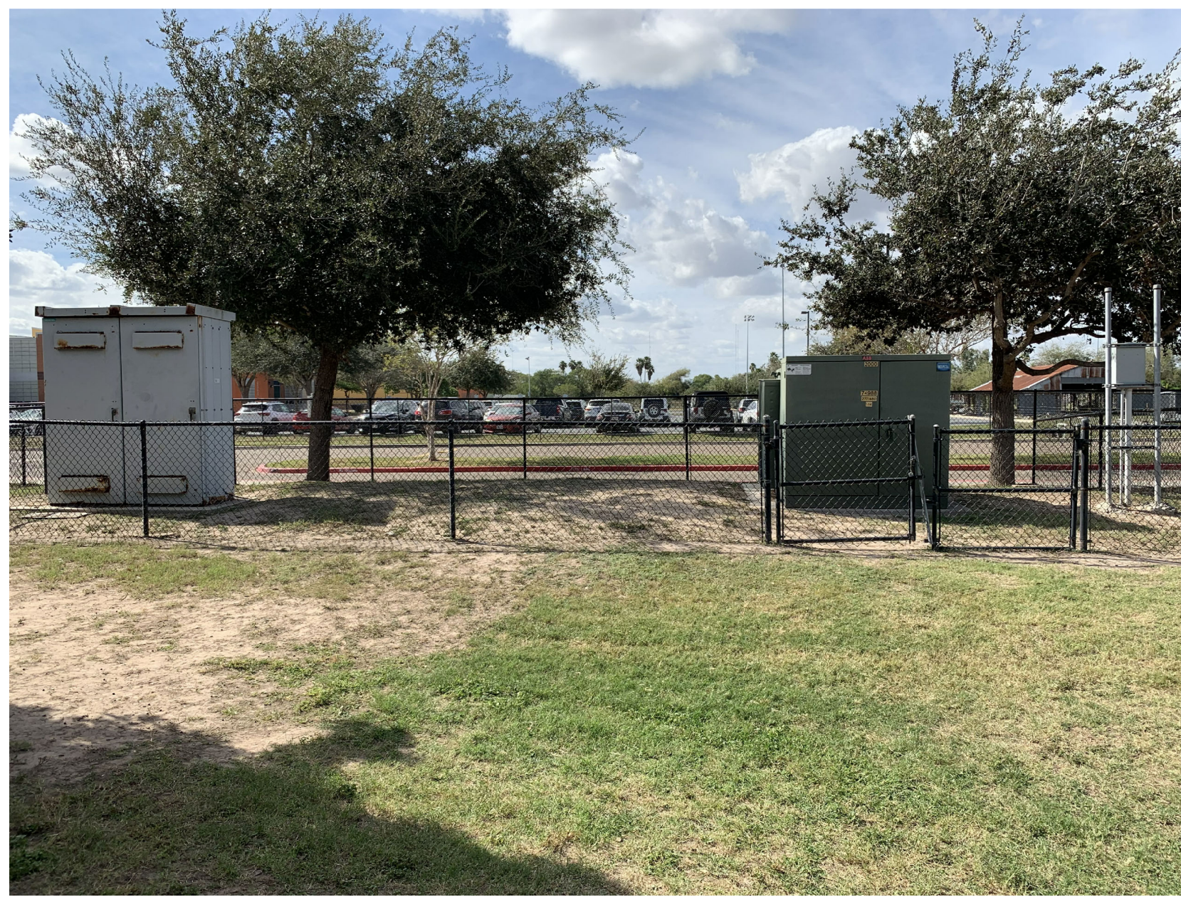
04 IMAGE EXISTING ELECTRICAL SERVICE ENTRANCE SCALE : NOT TO SCALE
