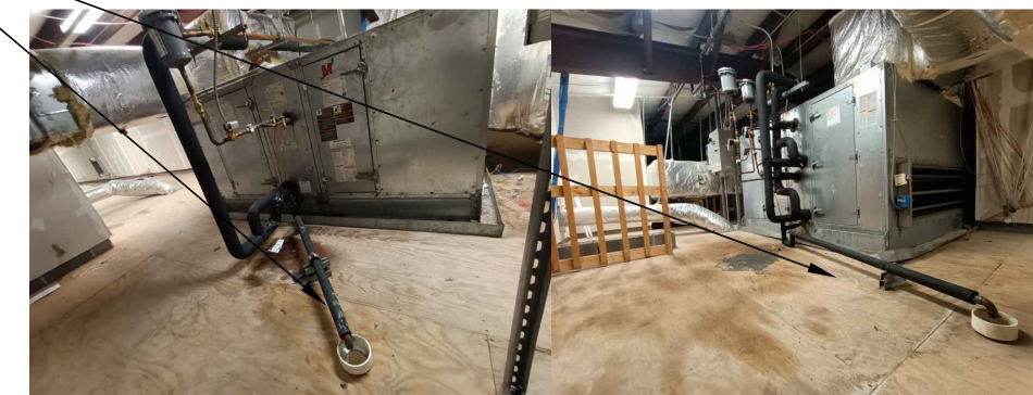
IDEA FRONTIER 03 EXISTING CONDITIONS AHU-3&4 (BUILDING C - MEZZANINE) SCALE: NOT TO SCALE
