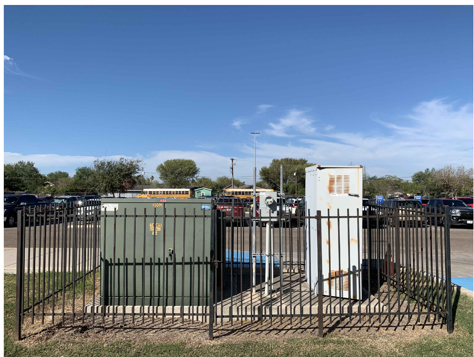
04 IMAGE EXISTING ELECTRICAL SERVICE ENTRANCE SCALE : NOT TO SCALE
